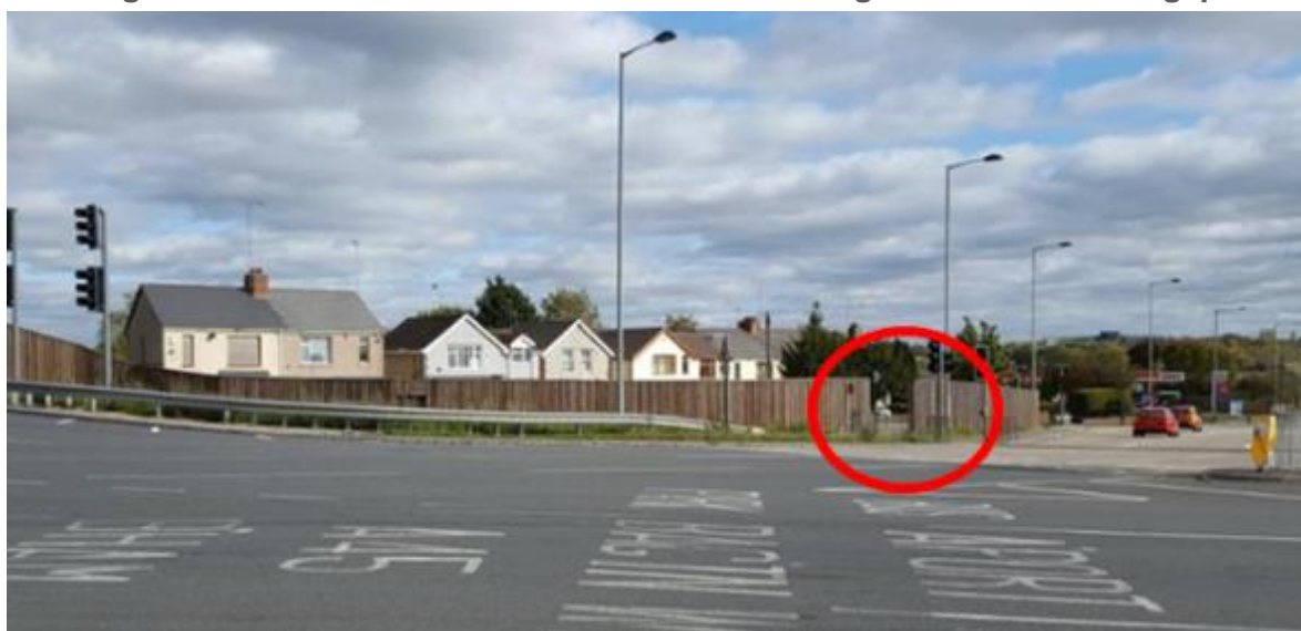
Figure 24: Noise barriers at London Road showing noise barrier with gap.
