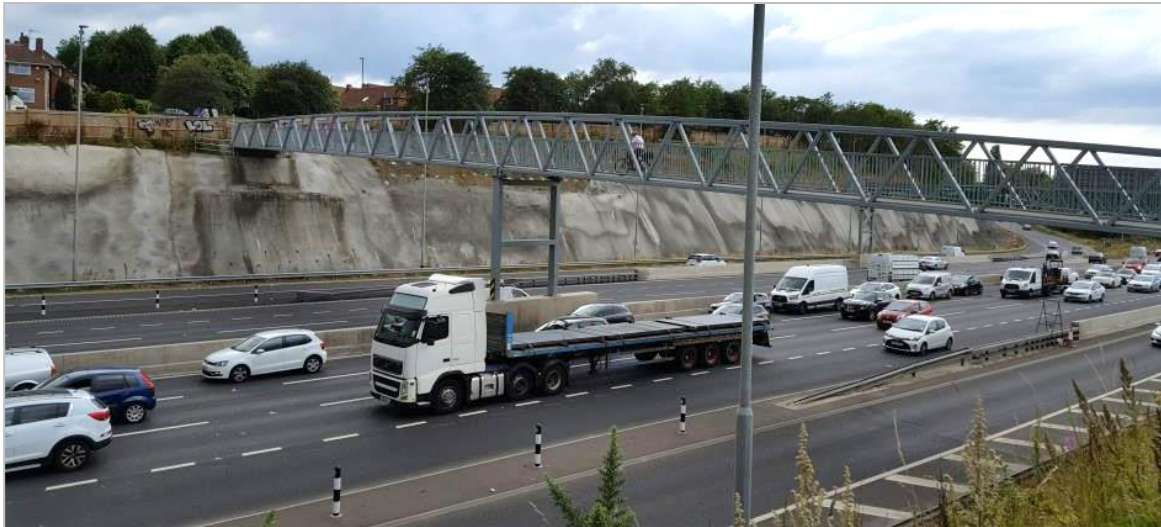
Figure 17 View of shotcrete at Gateshead Quays and replacement Chiltern Gardens footbridge cycleway
